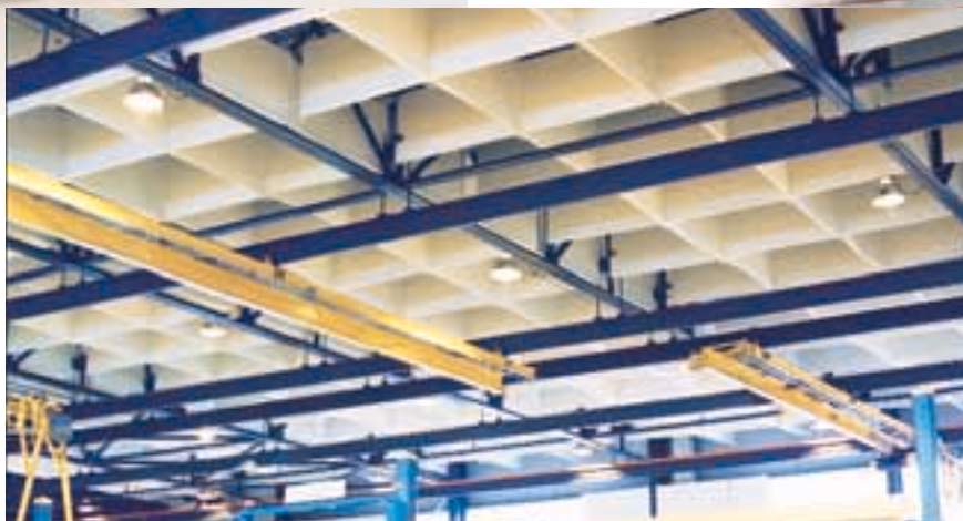
Baffelabsorber in Montagehalle Fa. Isofab Inc./Kanada
